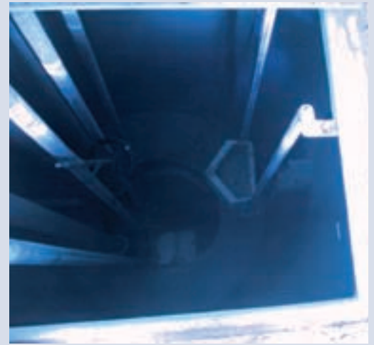
Grundfos supplied a complete solution, including all electrical and automation systems.
